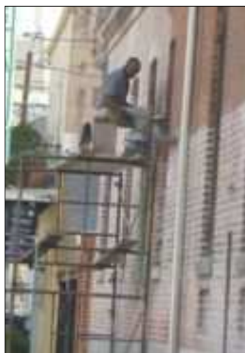
Master craftsman and historic masonry expert Teddy Pierre repoints a brick wall on a property that benefited from the Historic Building Recovery Grant program in New Orleans' Faubourg Marigny.
