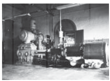
Shreveport's McNeil Street Pumping Station is listed on the Register under Criterion C in the area of engineering because it documents the technological evolution of a late-19th-early-20th-century waterworks.
